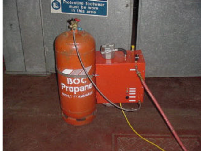
Figure 3 Shows a typical propane and oxygen supply system for flame spray process
