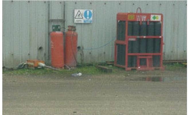
Figure 2 Shows a typical propane and oxygen supply system for flame spray process
